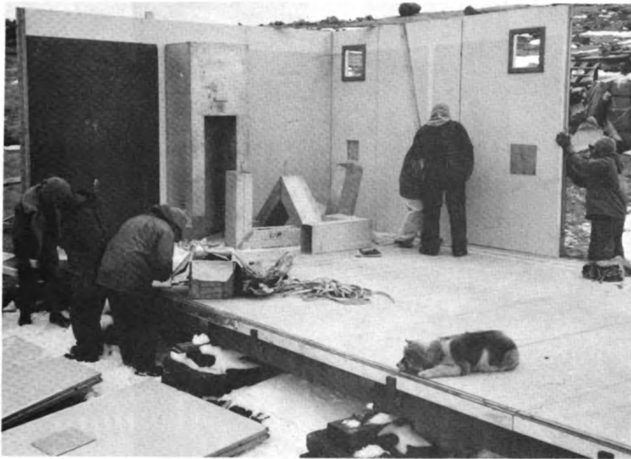
Standard sleeping hut during erection showing the heating-stove recess and hot air ducting.
